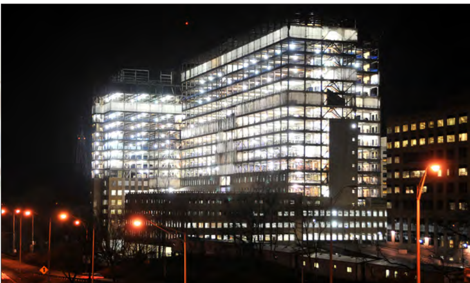
March 2010. The structural steel has been completed and work on the south garage has started. This is an example of the contractor working full crews on nights and weekends to ensure on-time completion. (Photo by Marc J. Barnes)
