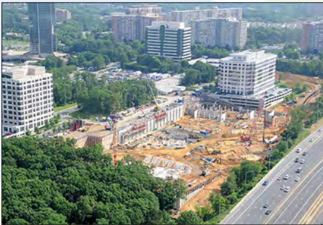
June 2009. The excavation has been completed. Pile driving has started and the first structural steel is being erected. (Photo by Marc J. Barnes)
